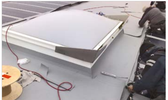
Fig. 14: The hand welding torch is used for the roof edges, which are difficult to reach.
